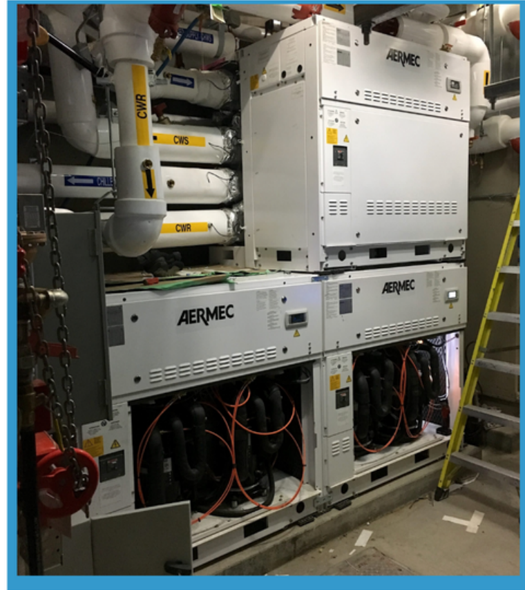
The Aermec WWM Modular Chiller units were placed side-by-side and stacked to fit within the equipment room's limited space.
